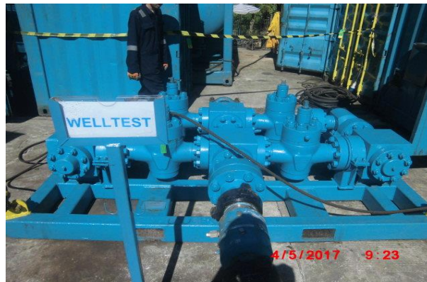
Gambar 1.4 Well Test Unit
