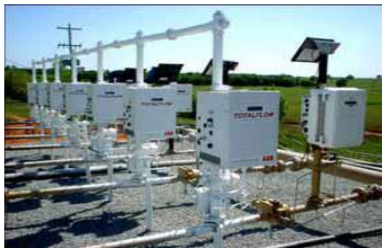
Gambar 3.6 Manifold (Havard Devold, 2013)
